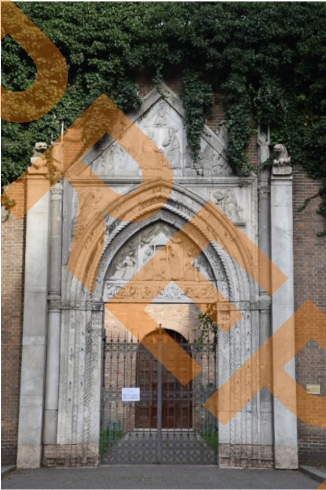
4: Gateway of San Giovanni Evangelista, Ravenna, condition after war damage and reconstruction of 1958. (Photo: author).
