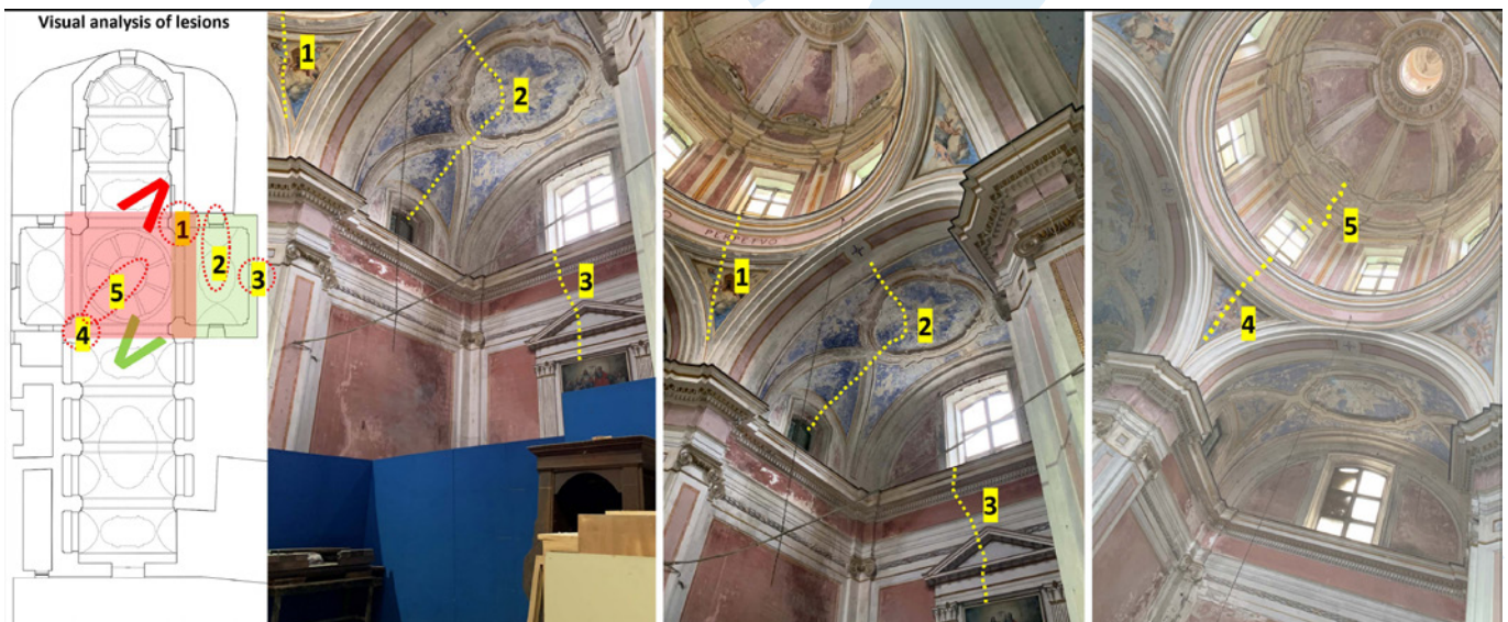
Fig. 2. Visual inspection of the crack pattern in the transept and dome area of the Church of Santa Maria della Vita, showing the spatial distribution and main orientations of the observed lesions on arches, vaults, pendentives, and the drum (prepared by R. Iaderosa).
